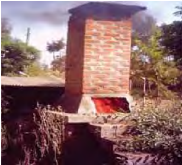
Figure 23.4 An incinerator used for healthcare waste. (Photo: Muluken Azage)
