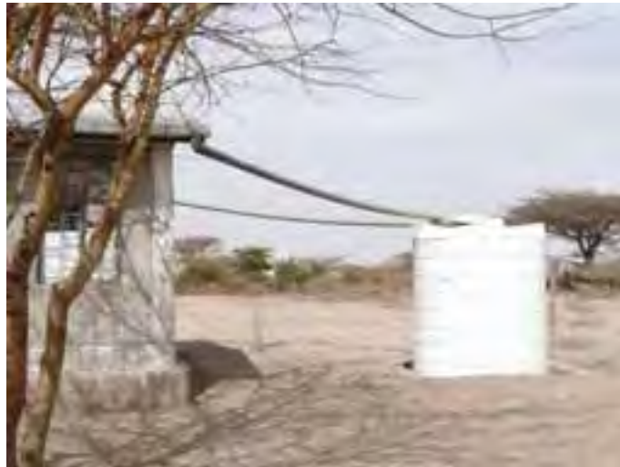
Figure 15.1 Rainwater is collected from the roof of this health centre and stored in a covered, watertight cistern. (Photo: Pam Furniss)
