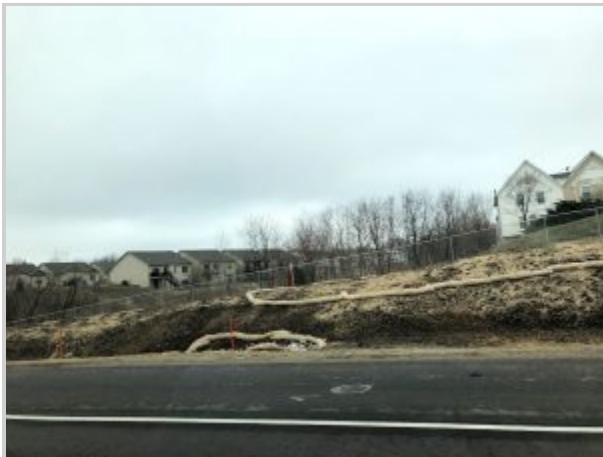
New construction is particularly sensitive to erosion, this disturbed shoulder off of I-35 near Ankeny is using a few techniques to control erosion-straw waddles and straw to help grass seed establishment. Photo Credit: Amber Anderson.
