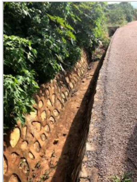
This road ditch in Uganda has complete covered the area water would run with cement and rocks so it cannot erode and undermine the road. Photo Credit: Amber Anderson.
