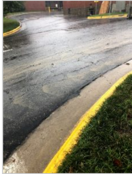
Runoff off of a construction site on ISU campus
