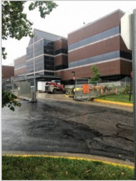
Runoff off of construction site on ISU campus
