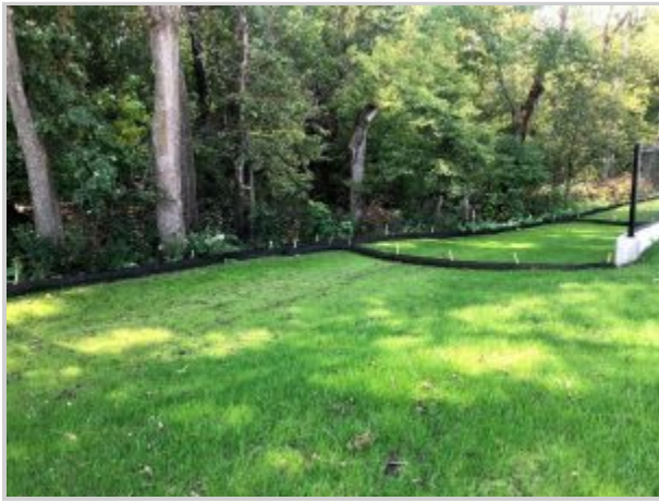
As the perennial cover of grass gets established next to the new Ames High School, these black strips are used to slow water and stop sediment moving down the hill. Photo credit: Amber Anderson.
