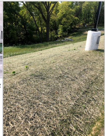
This reinforced mat is being used on a steeper part of the landscape while grass is being established that will stabilize the area for the long term. Photo credit Amber Anderson
