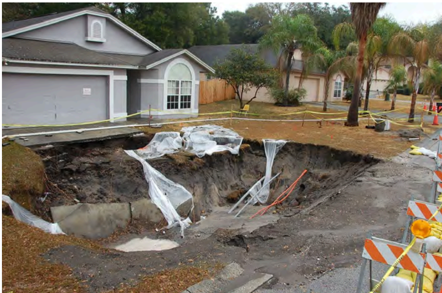
Figure 11.39: This sinkhole from collapse of surface into a underground cavern appeared in the front yard of this home in Florida.
