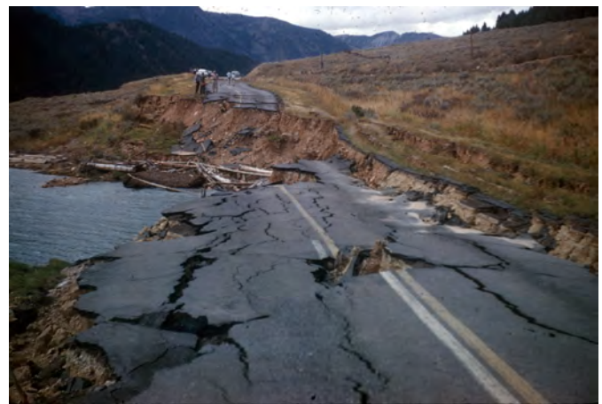
Figure 10.8: Road damage from the August 1959 Hebgen Lake (Montana-Yellowstone) earthquake.
