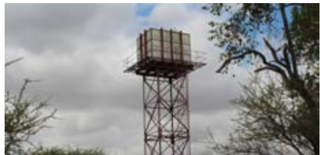
Water tank for village water supply © G. Matswiri
