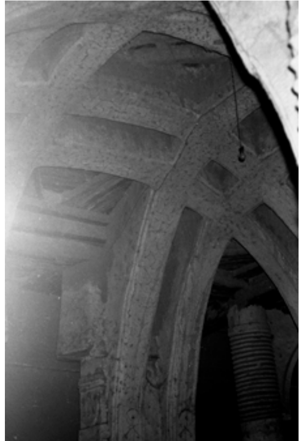
FIG. 672. Interior of the Zaria Friday Mosque showing how the double arches meet to form an imitative vault. Palm wood is laid in patterns to fill the interstices. Mallam Mikaila, Hausa male architect, Zaria, Nigeria, 1830s-40s. Photo by Hamo Sassoon, 1930s-1970s. Pitt Rivers Museum, 2005.113.937. Creative Commons CC BY-NC-ND 4.0.
