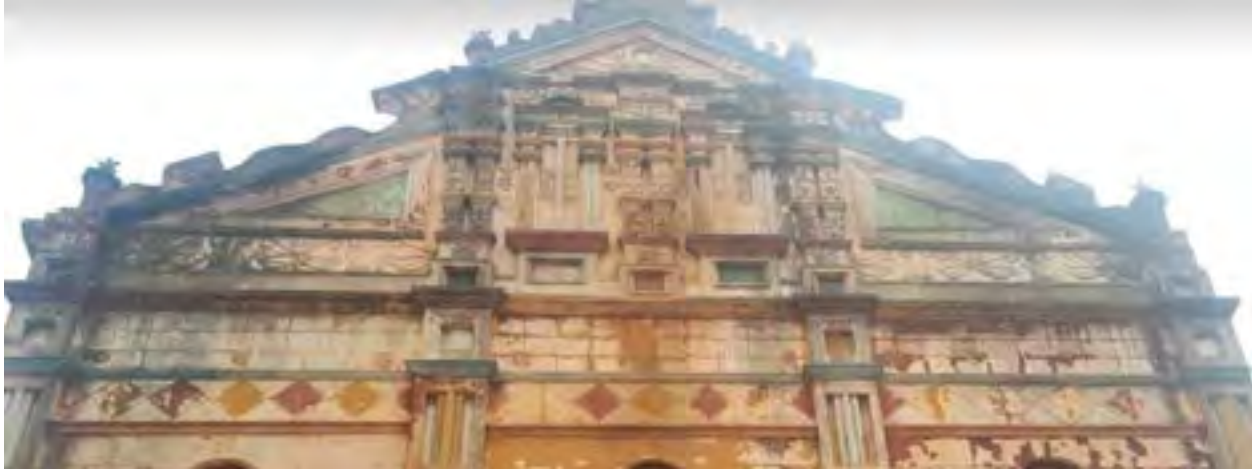
FIG. 663. The upper section of the rear facade of Porto-Novo's Great Mosque includes numerous floral plaster surface reliefs. Photo by Annabelle Bennetier for Google Earth, 2018.
